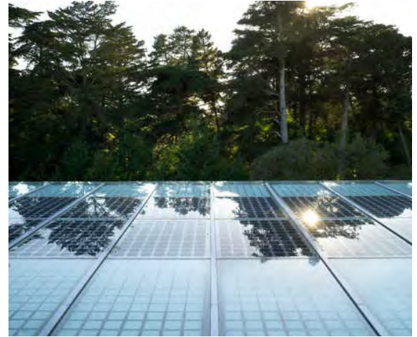
Clean energy generation for the campus is a key component to meeting environmental goals.
